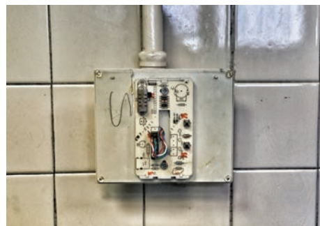
Exposed wall switch in a student bathroom, Elementary School No. 20, Paterson.
