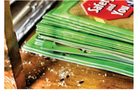
Mouse droppings in an in-use classroom, Elementary School No. 20, Paterson.
