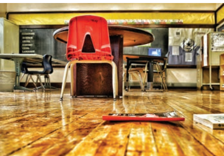
Warped floorboards in an in-use classroom, Elementary School No. 20, Paterson.
